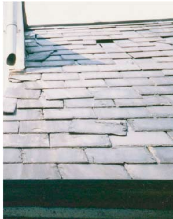
Loose tiles pose a threat to passers by.
