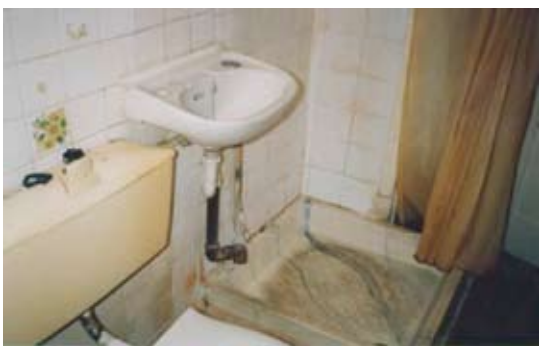
This sink has no direct supply of either hot or cold water which is unacceptable.
