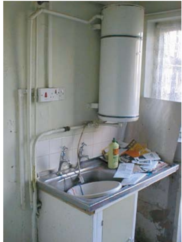
Old lead pipework may pose a threat
