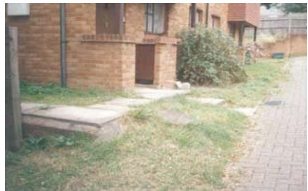
Uneven paving slabs may pose a significant hazard
