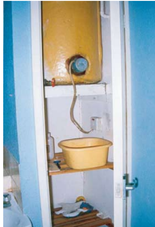
This continuous leak is an electrical hazard.
