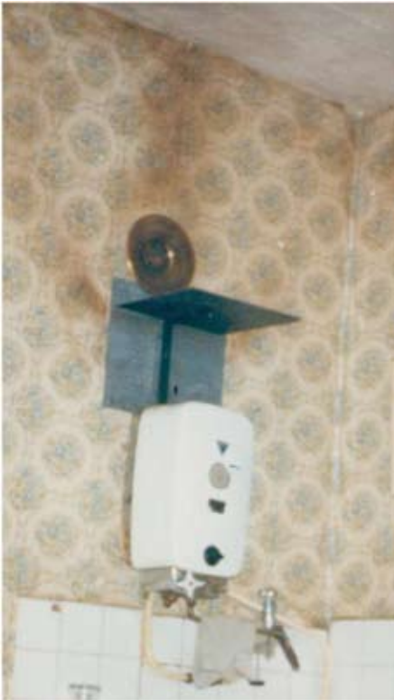
This water heater doesn't have adequate ventilation which can be seen by the damage to the wall and ceiling
