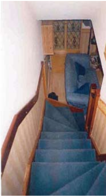
This staircase does not have any handrails which poses a threat to safety, particularly to older people.
