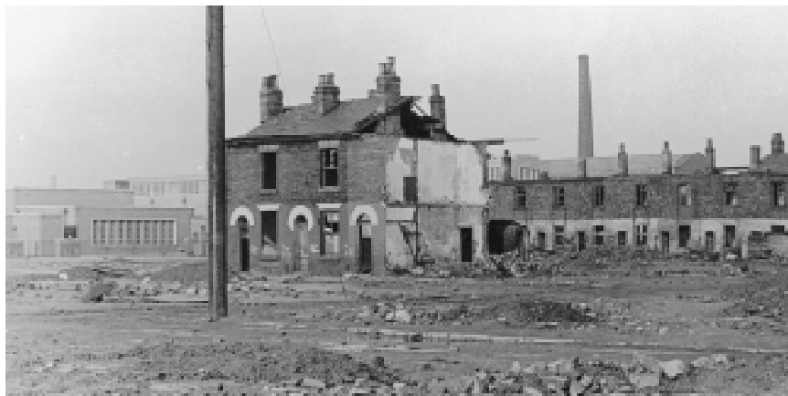
Demolition – Clarendon School can be seen in the background. (Photo taken and donated by Ernest Jones)
