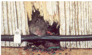
Gnawed electrical lead
