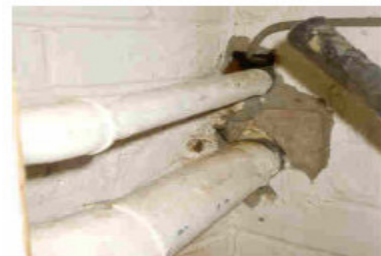
Holes around pipes
